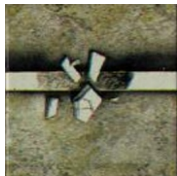
Breached Wall Tile
